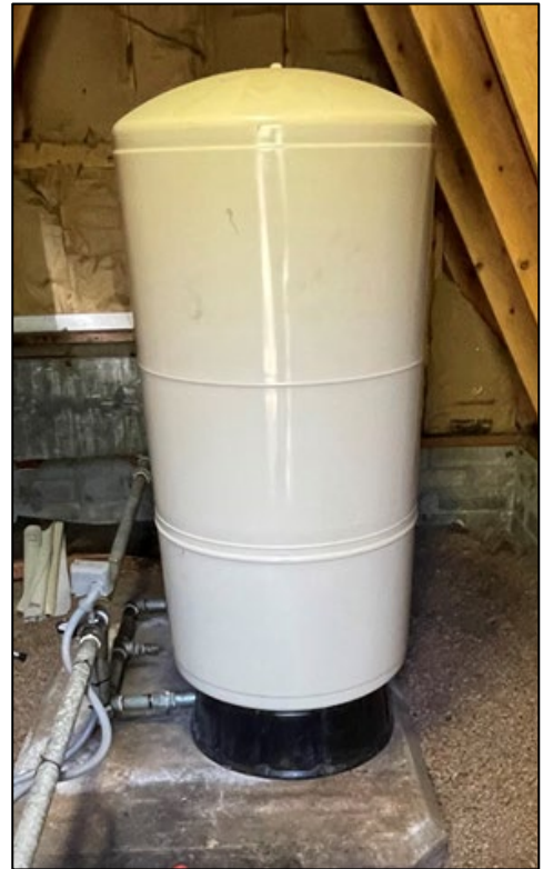
Bladder Tank at VG2 Pump House
