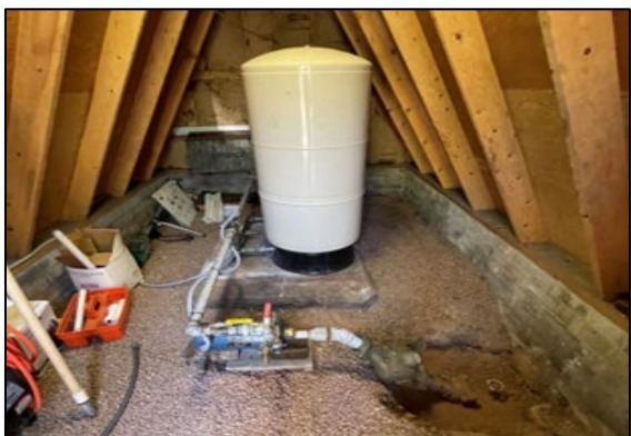
VG2 Pump & Bladder Tank
