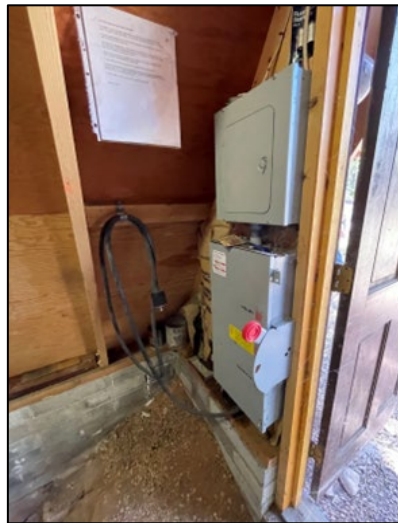
Electrical Controls at VG2
