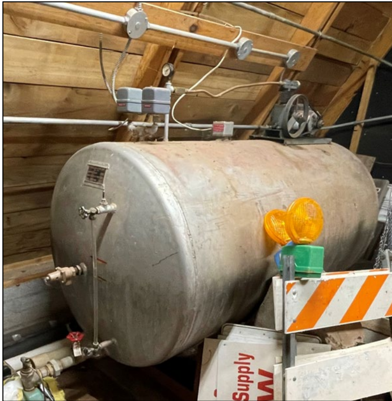
HP Tank at VG1 Pump House
