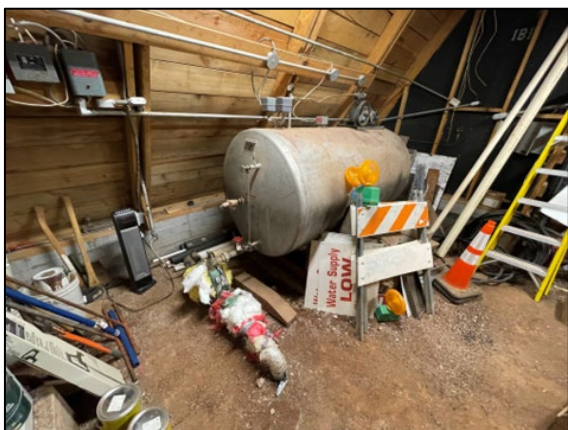
VG1 Pump & HP Tank
