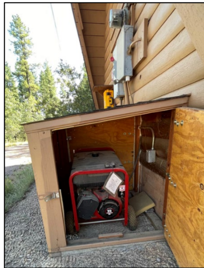
Mobile Emergency Generator stored at VG1
